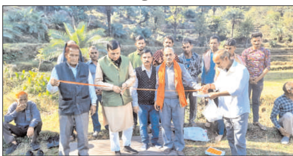
DDC, Kathua, Col Mahan Singh (Retd.) starting construction of Sump Collection Tank.
