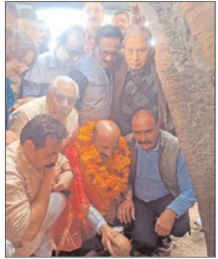
MLA Mohan Lal laying the foundation stone for new passenger shed at Akhnoor.
