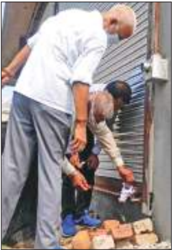
JDA employees sealing illegal construction.
